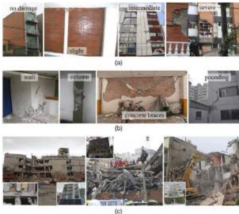
Figure 7. Examples of observed damages: (a) nonstructural damage, (b) structural damage, and (c) collapses.
